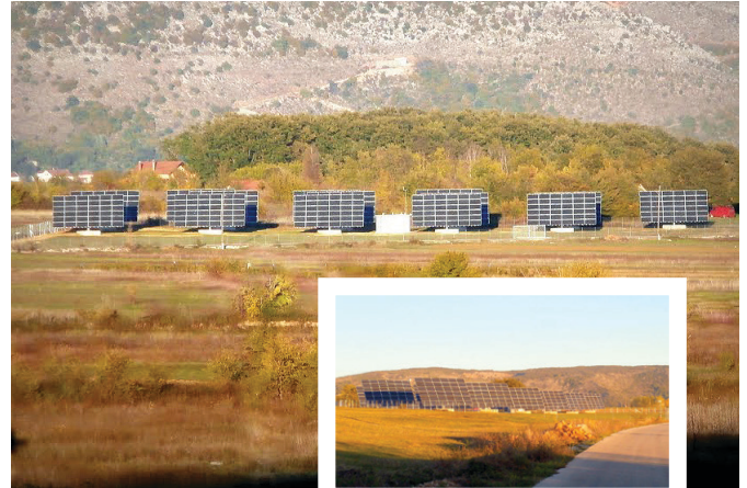
Drinovci – solar photovoltaic power plant KRENICA 1
